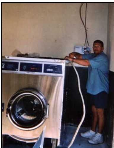
Volunteer handyman André Ouellette setting up the laundry machine's electrical and plumbing connections.
