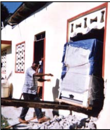
One of the walls at the Brenda Strafford Hospital had to be partially torn down and rebuilt to allow a donated laundry machine to be installed.
